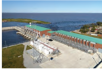
Water pump stations (completed in 2017)
